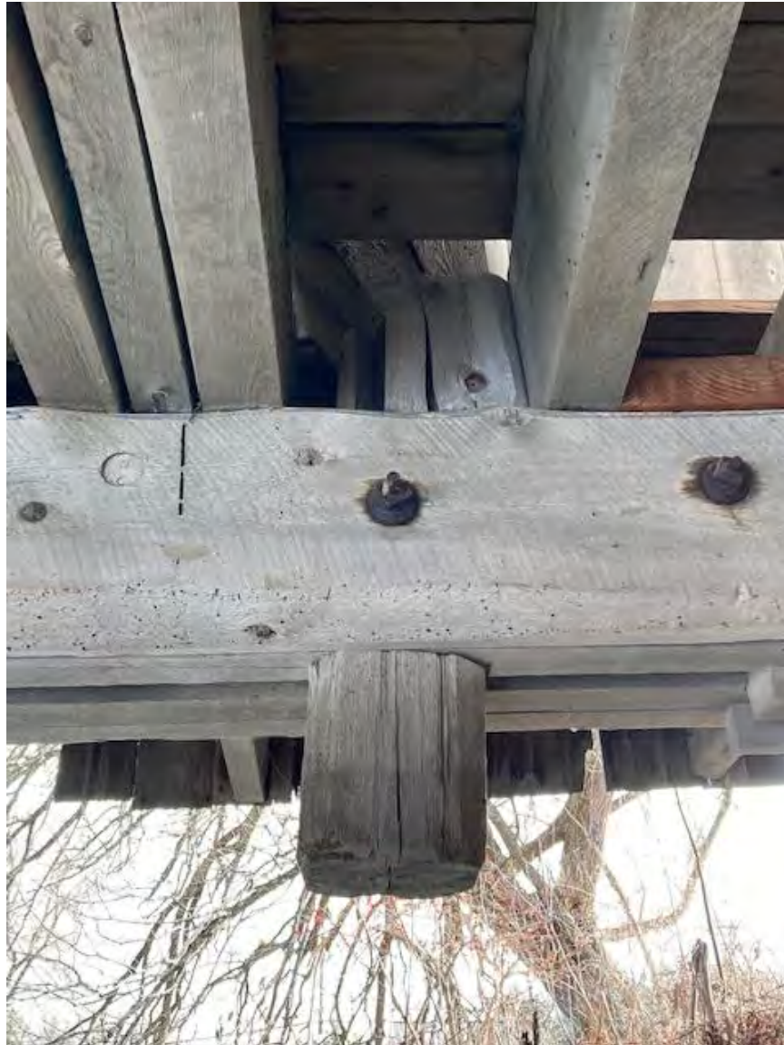
Sanborn Bridge: broken and displaced post bottom near abutment
